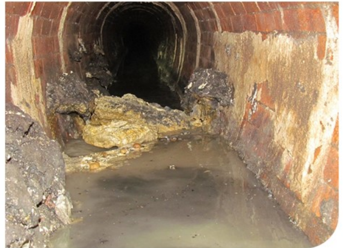
A giant 30-tonne fatberg was cleared from a sewer near the Shard in London last year
